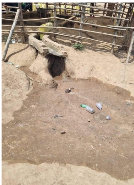
The drainage is creating a source of contamination.
